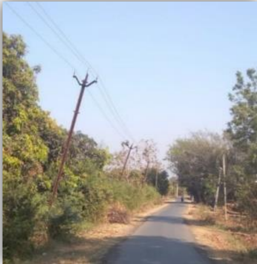
Fig. 4.14 Electric transformer and pole (Kewada Village)
